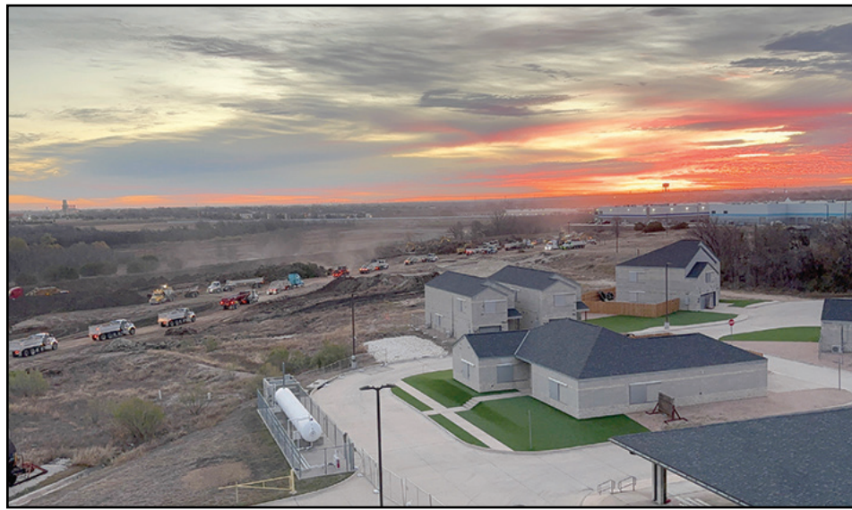
AP starts construction on Round Rock Public Safety Training Center expansion photo credit: City of Round Rock
