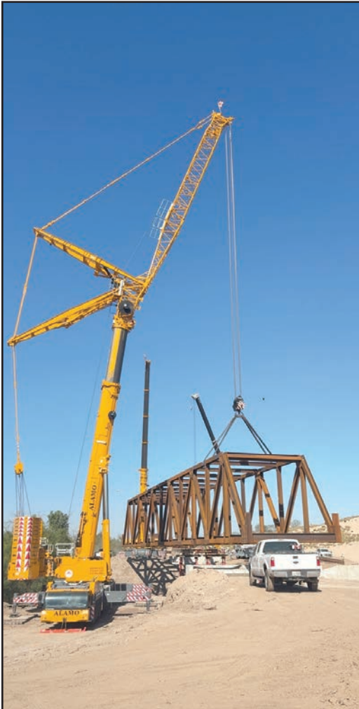
Alamo Crane's LTM 1650-8.1, 770-ton Liebherr crane team picking a 120-ft. steel truss bridge with Alamo Crane's LTM 1300-6.2, 360-ton Liebherr crane.
